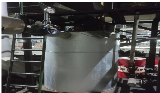
Gambar 2. Thermal oil heater
