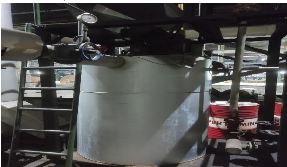
Gambar 2. Thermal oil heater
