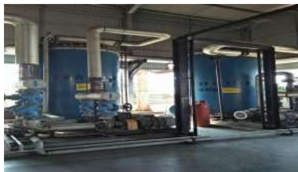
Gambar 1. Thermal oil heater
