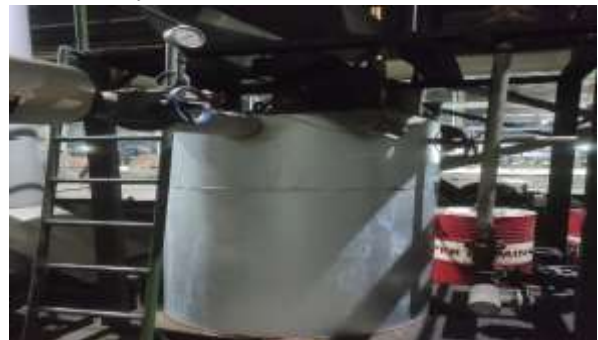
Gambar 2. Thermal oil heater
